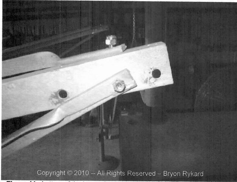
Figure 11: bottom of the Lower Angle Iron "X" bracing attached to the tower.
